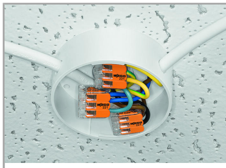
Lighting distribution in ceiling canopy
