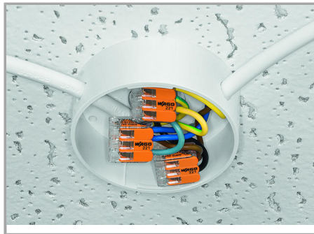
Lighting distribution in ceiling canopy
