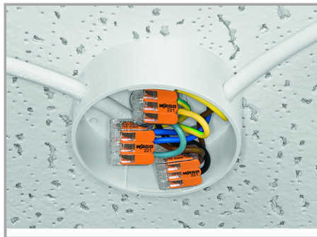
Lighting distribution in ceiling canopy
