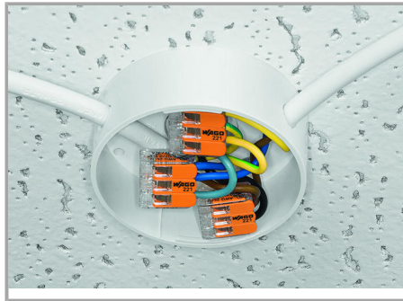
Lighting distribution in ceiling canopy
