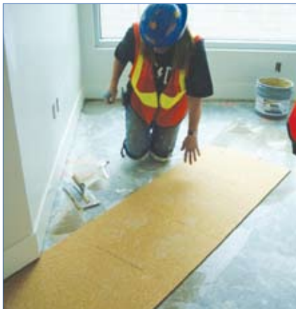
Sheets of AcoustiCORK CRC950, a new 3/8" thick Cork & Rubber composite sheet material being applied to a concrete subfloor. Ceramic tiles will then be installed over the underlayment.
