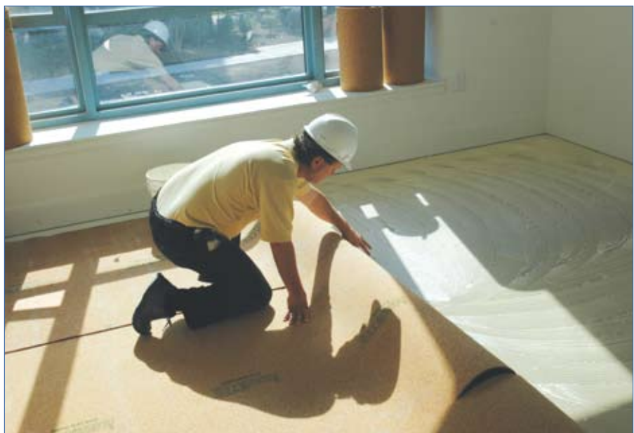
Installing 6mm AcoustiCORK Underlayment rolls in a glued down engineered wood floor application over a concrete subfloor.
